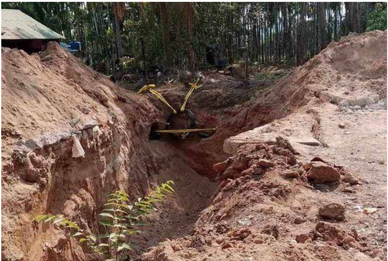
Figure 4: Road between Kan Pauk and Na Bu Lel destroyed by the Myanmar military, April 2023. Photo: Local
